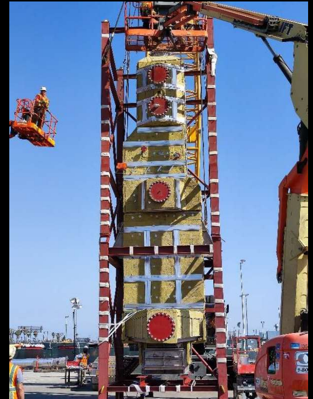
Installation in Long Beach, CA
